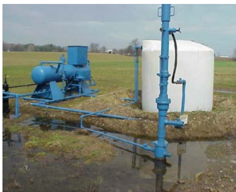
Photo 6. Gas well with new plastic brine tank in Town of Java, Wyoming County. Rustproof tanks can help prevent leaks.
