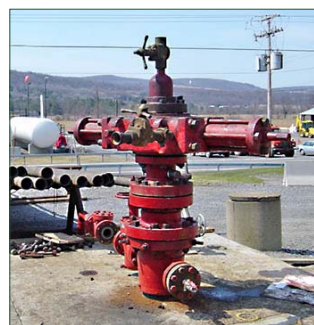
Well at New York LPG's Underground Storage facility in Cortland County.
